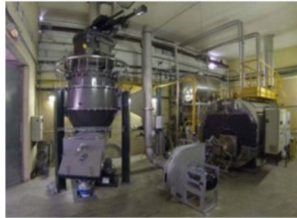
2 MW capacity Syngas from wood chips
